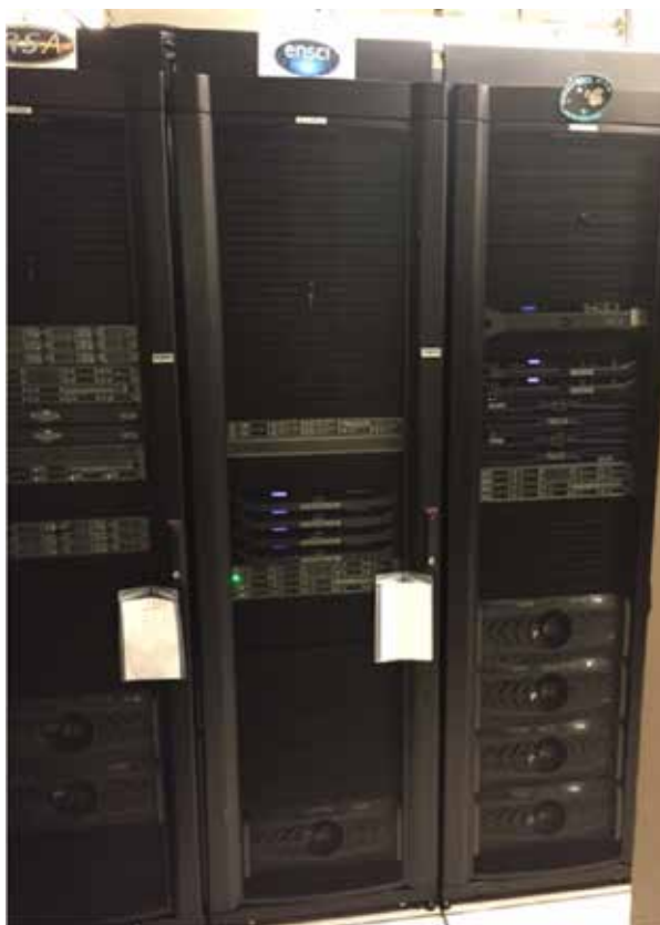
The first rack of dedicated SDC-US equipment in the IPAC data center.
